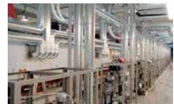
Thermal oil control circuits
